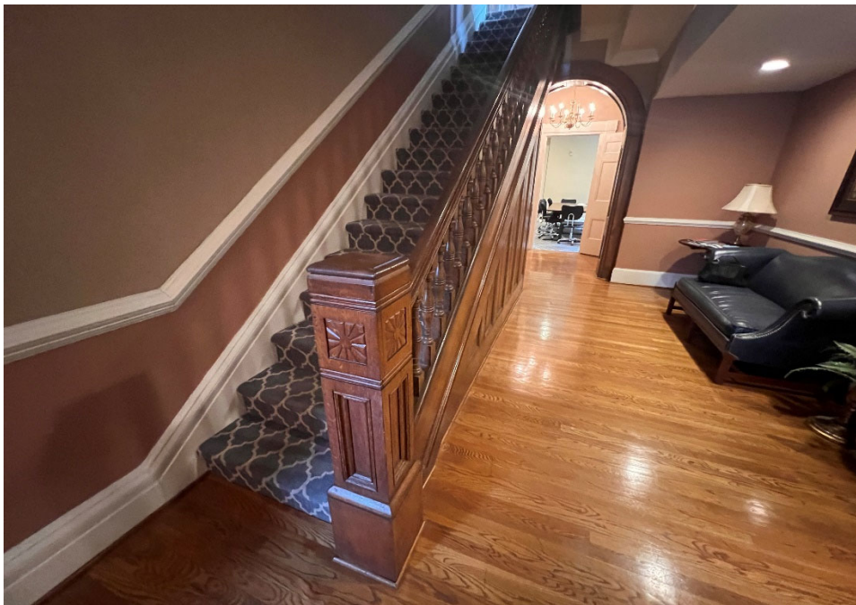
The structure around the main staircase has slightly deflected.
