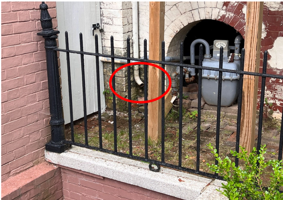
The neighbors gutter downspout is discharging close to the building and the nearby retaining wall.
