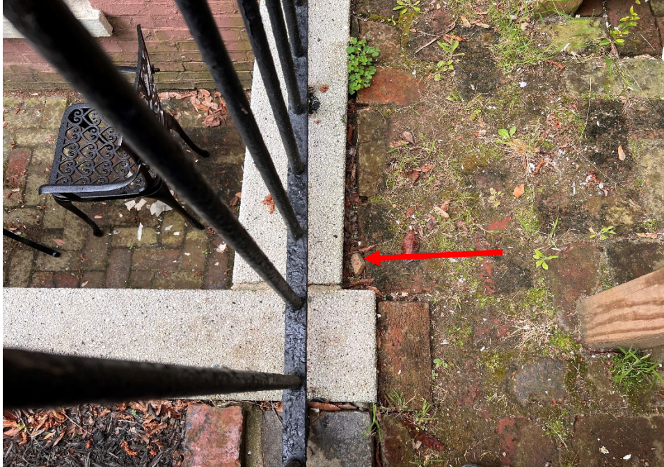
The retaining wall has been pushed inward several inches.
