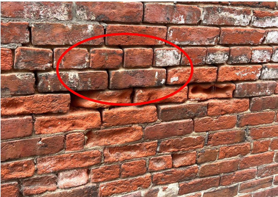
Mortar is deteriorated or missing in several areas around the building.
