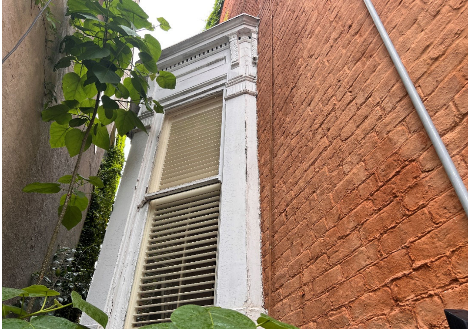
The owners would like to remove this bay window. Vegetation grows on the masonry behind the window.
