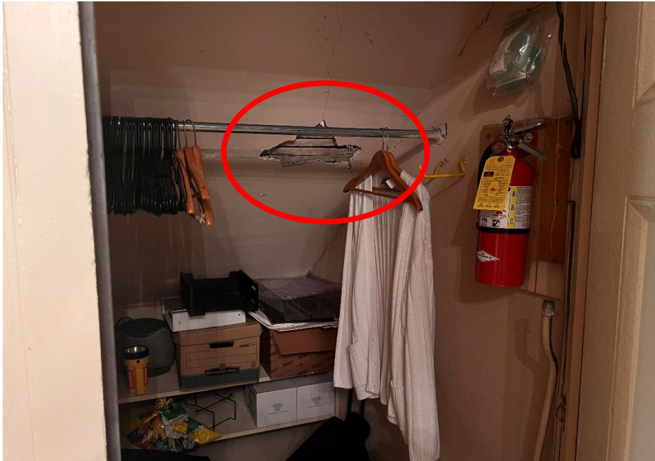
Plaster has fallen off the lathe work in the closet under the stairs.
