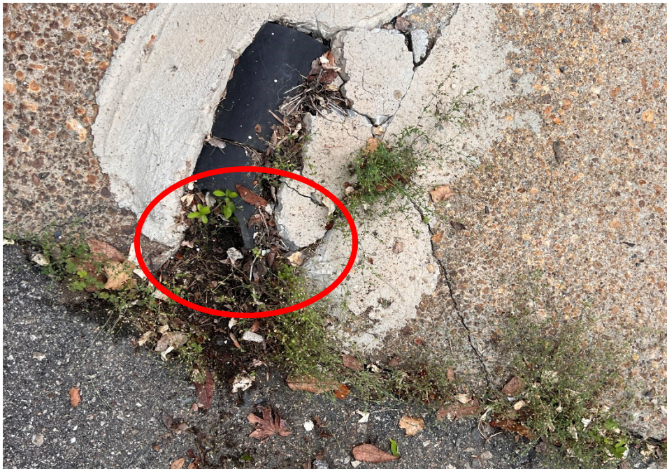
This downspout is routed to the rear alley, but it appears clogged with debris.
