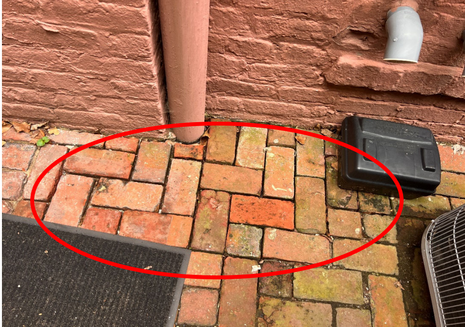
The lack of mortar or earth around the base of one downspout suggest that water overflows in the area.
