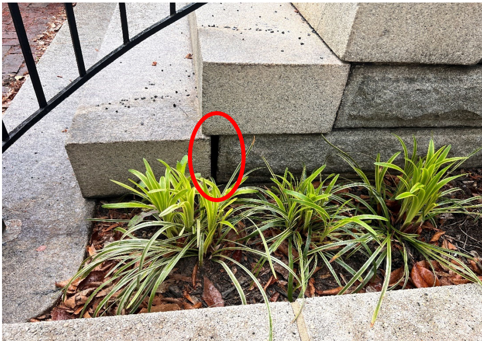
Gaps and voids have formed on the granite staircase.
