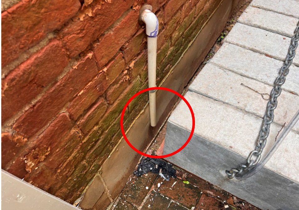
Several HVAC condensate lines are discharging at the base of the buildings foundation.
