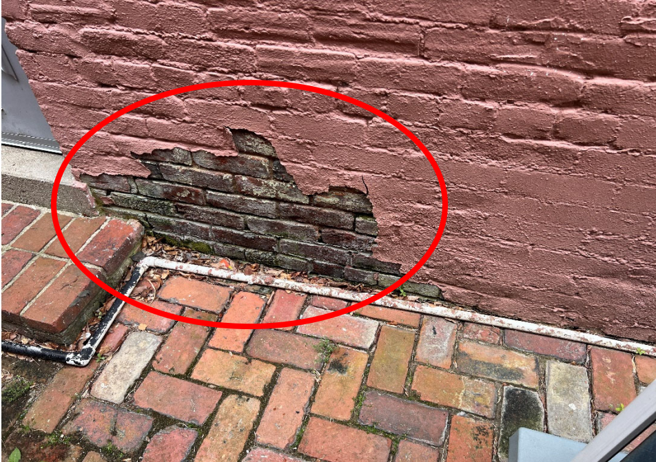
Paint spalling and flaking off near the earth line suggest that water may be present inside the wall.
